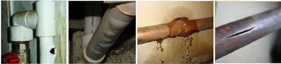
Fig. 1. Examples of damage in piping systems due to hydraulic shock
